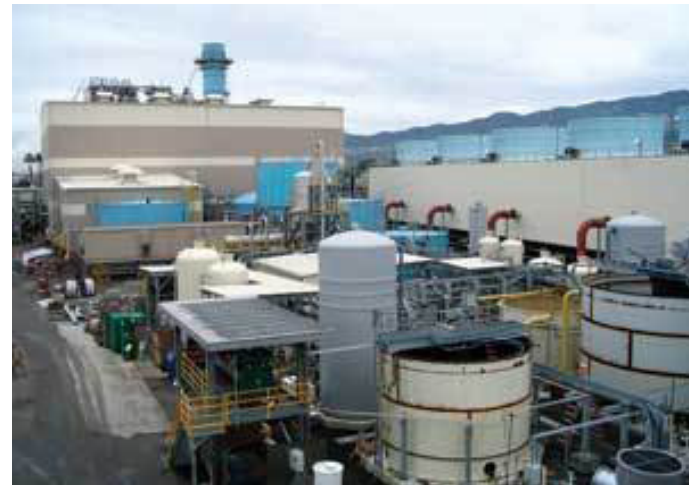
Make Up Water Treatment Plant
