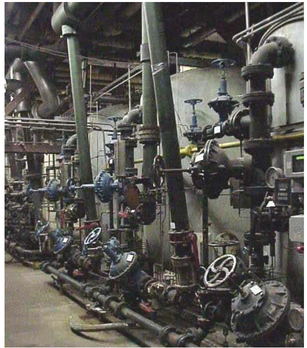
Typical Make-Up Water Treatment plant showing Ion Exchange Beds along with make up water inlet and outlet manifolds
